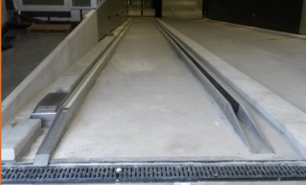
Location: Rotterdam, Holland Installed: September 2015 Length: 69' [21 m] Indoor
