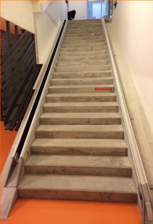
Location: the Hague, Holland Installed: October 2015 Length: 27.5' [8.4 m] Indoor
