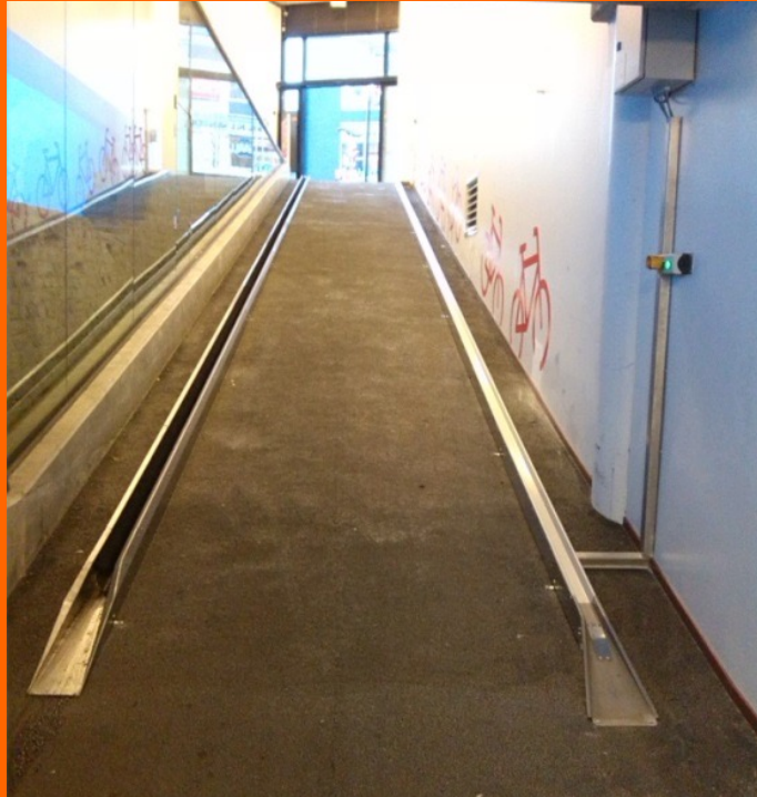
Location: Utrecht, Holland Installed: December 2014 Length: 59' [18 m] Indoor
